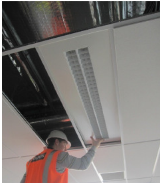
Figure 8: Unsecured recessed luminaires
