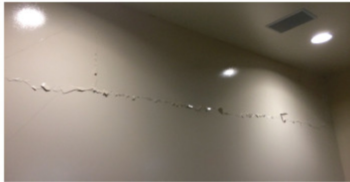
Figure 12: Cracked gypsum board wall in hospital
