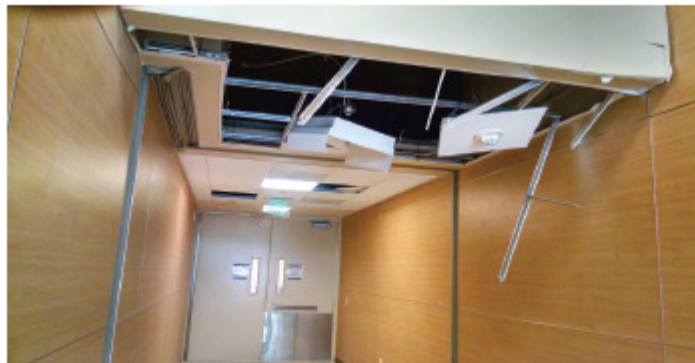
Figure 13: Ceiling damage in hospital corridor link
